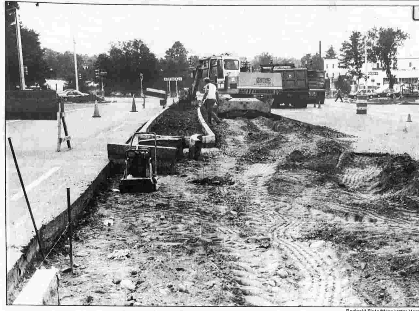
ONE MORE TIME — Rich Prisle, a foreman for Tilon Tomasso of New Britain checks work being done on the intersection of Buckland Road and Tolland Turnpike Monday. The state recently completed work on the intersection, but it had to be widened under State Traffic Commission requirements for road improvements associated with the Pavilions at Buckland Hills.
